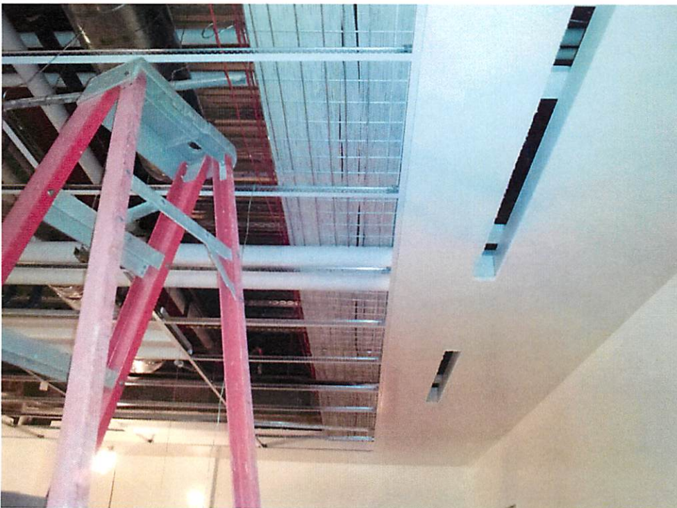
Fiber and Copper Data Cable Tray – Science Building, 1 st Floor Classroom
