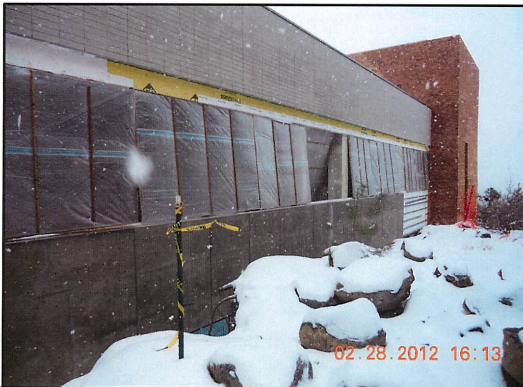
North Elevation: Wood shingle work complete. Window system about to be re-installed.
