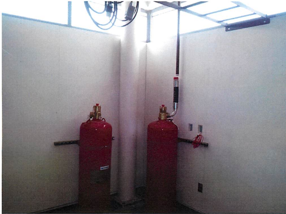
Novec Clean Agent Fire Suppression System – Health Careers, MDF
