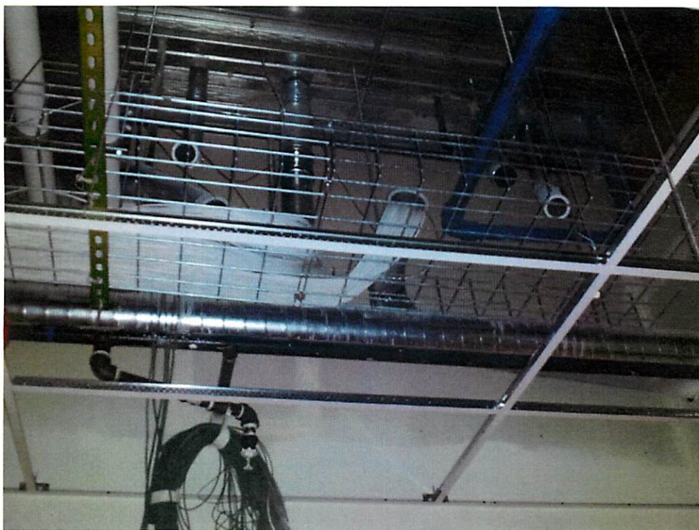
Cable Pathway Conduits – Science Building, 1 st to 2 nd Floor
