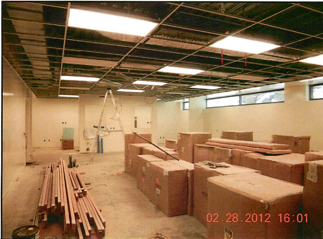
Human Biology Lab 120, grid and lighting in place. Ceiling tile install next week.
