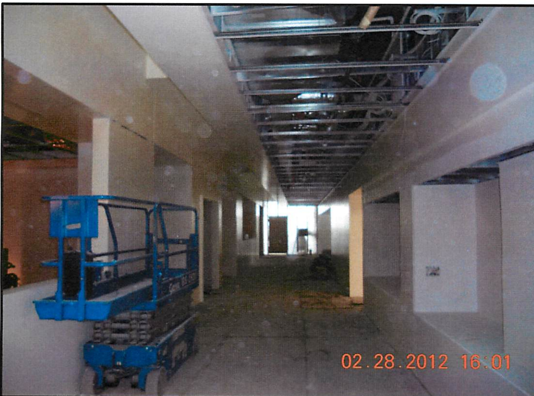
Hallway between Biology Labs painted with grid ceiling installed. Ready for diffusers and lighting.
