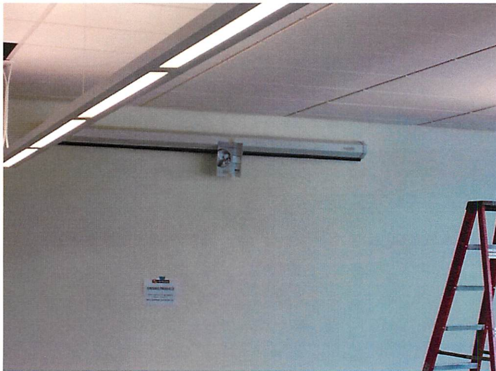
Typical Projection Screen Install – Health Careers, 2 nd Floor
