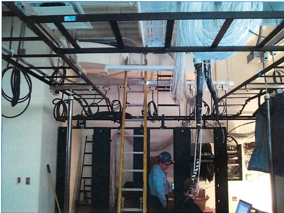
Switch Racks & Cable Ladder – Health Careers, MDF
