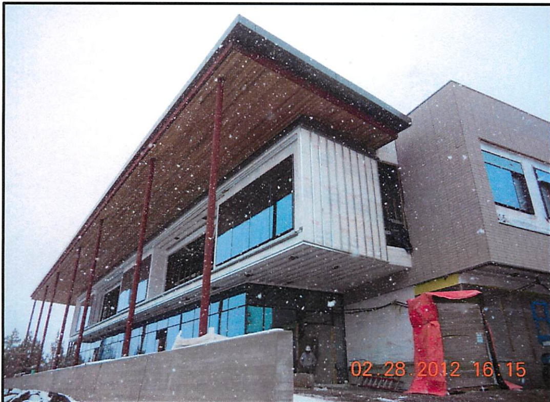
West Elevation glazing and wood soffit work in progress. Composite metal panel beginning.
