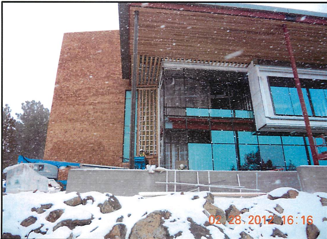
Northwest corner of building. Horizontal wood siding install at bathroom exterior wall.
