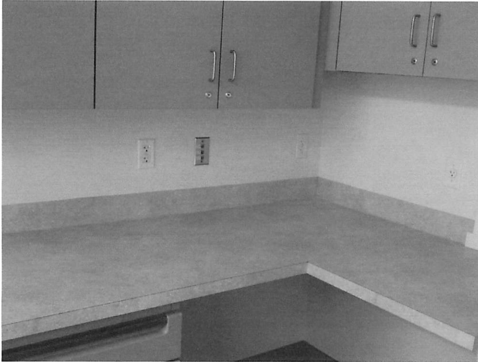
Typical Data Jack Installation – Pharmacy Lab
