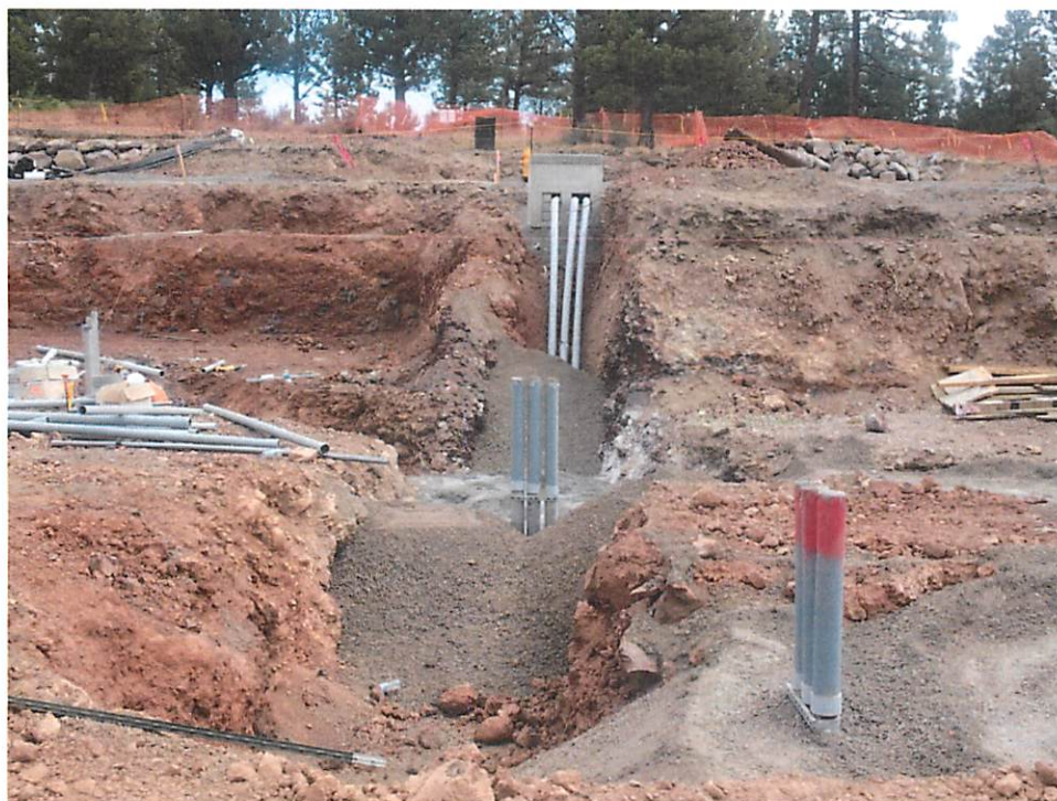
Communications Conduit – Vault to Primary MDF
