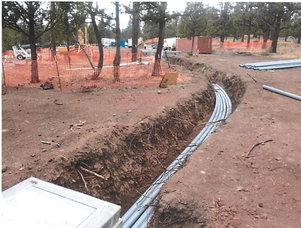
Communications Conduit – Low-Voltage Trench
