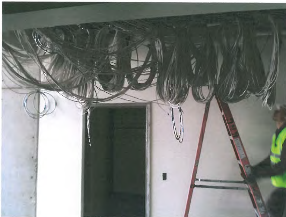
Second Floor Data Pulls – Outside MDF
