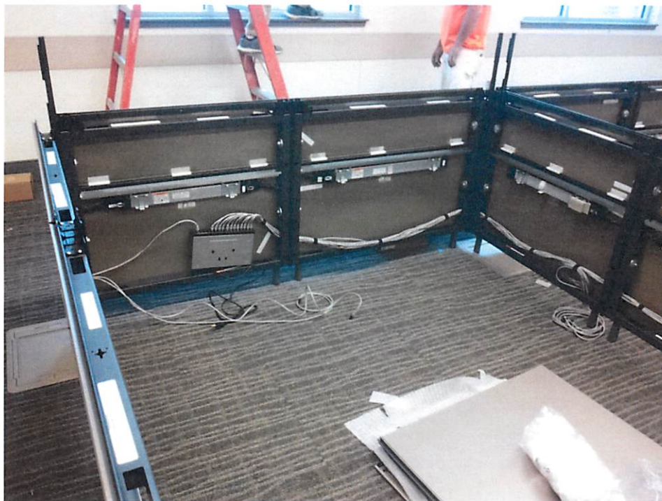
Wiring furniture for network connectivity – Computer Classroom 137
