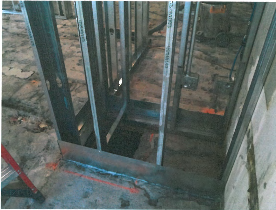
Low-voltage chase – Second Floor, Grandview
