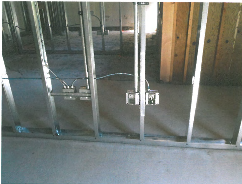
Typical low-voltage box and conduit – Office Area, Grandview
