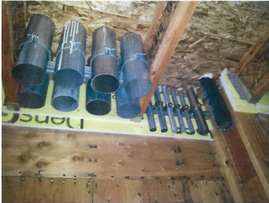
Low-Voltage Sleeves – Residence Hall, Middle Bar
