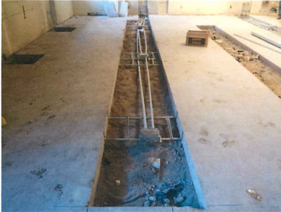
Power & Data Floorboxes – Computer Lab, Ochoco remodel
