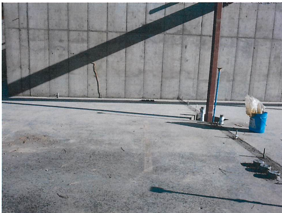
MDF floor and conduit entrances – Upper Bar
