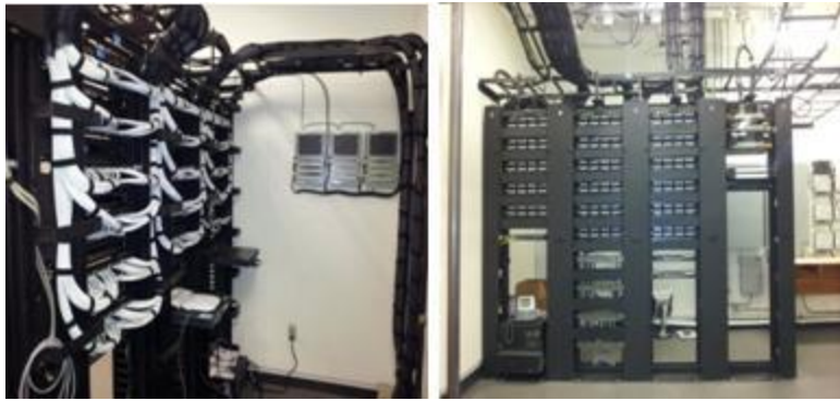
New Data Center equipment to manage the 45 miles of new data cables installed in just the Science and Health Careers Bldgs.
